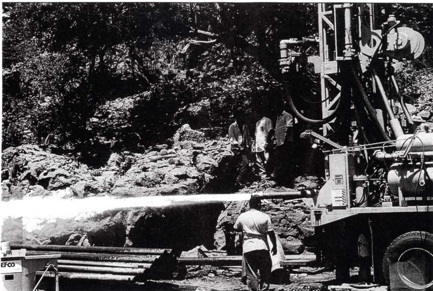
Bedrock test well drilling in Guarabal, Venezuela. Two test wells were drilled which produced a combined yield of more than 600 gallons per minute.
